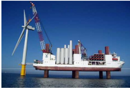
Turbine Installation Vehicle
