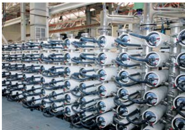
Orange County Water District
